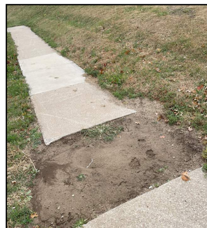
Existing/Current: Missing Sidewalk Section
